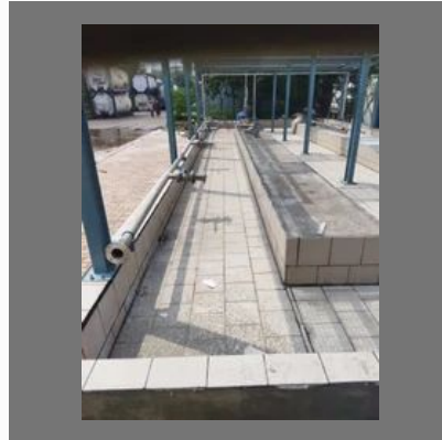
Acid Resistant Tile Lining Service
